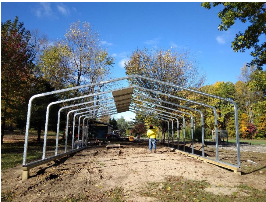
Work is progressing on the new picnic shelter. The foundation beams and steel framing up in place. The roof sheeting has started.
