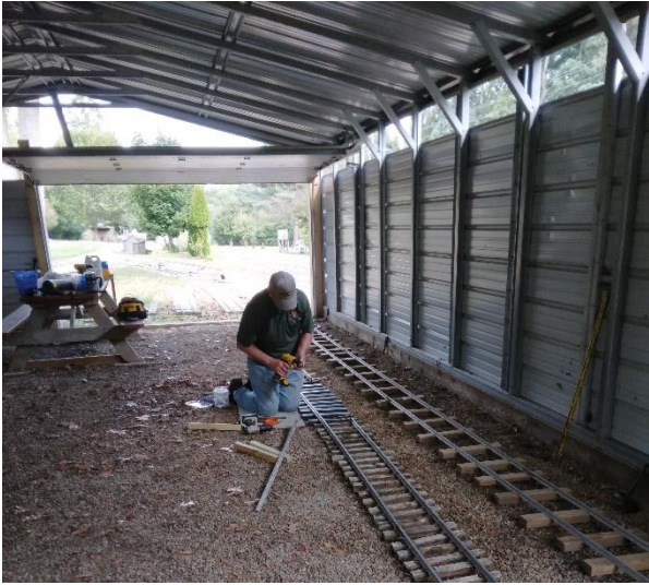
Dan Bockheim the clubs tireless track worker laying track in the new barn.
