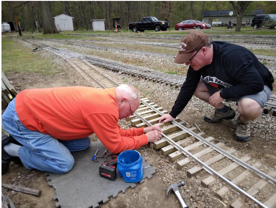
Mean while back at the ranch Jim Trimstra and Bret Pitchard were making up rail joints on the new ballast hopper siding.
